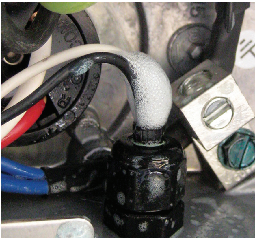
FIG. 7. A leak path can exist in a sealed luminaire.
