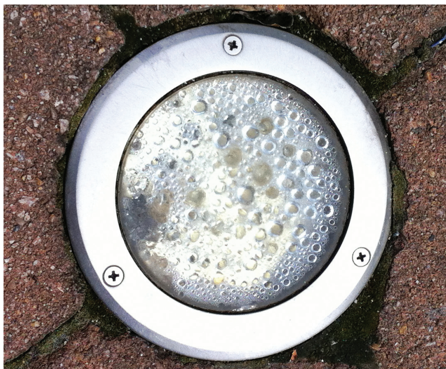
FIG. 5. Condensation inside an LED luminaire limits performance.
