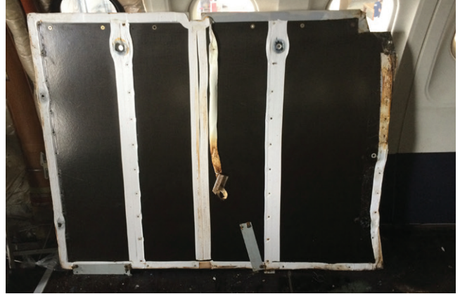
Figure 4: Material torn away from fastener holes and corners, separating from panel, and gaps in sealant
