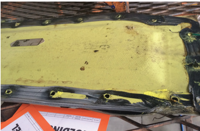
Figure 2: Material torn away from fastener holes and corners, excessively compressed (black), and separating from panel
