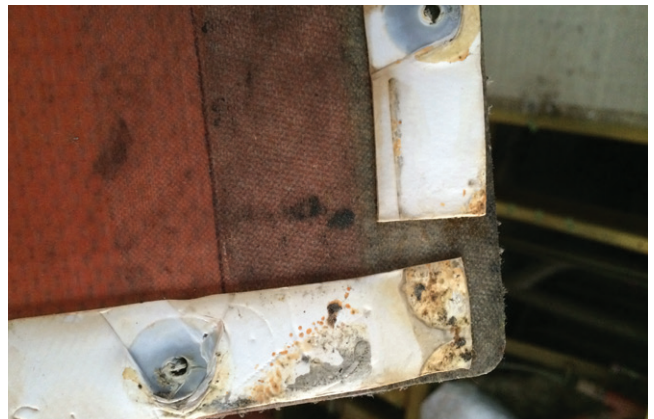
Figure 5: Improper corner overlap and gap between materials
