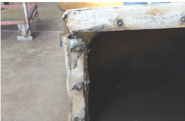
Figure 3: Material excessively compressed and worn
